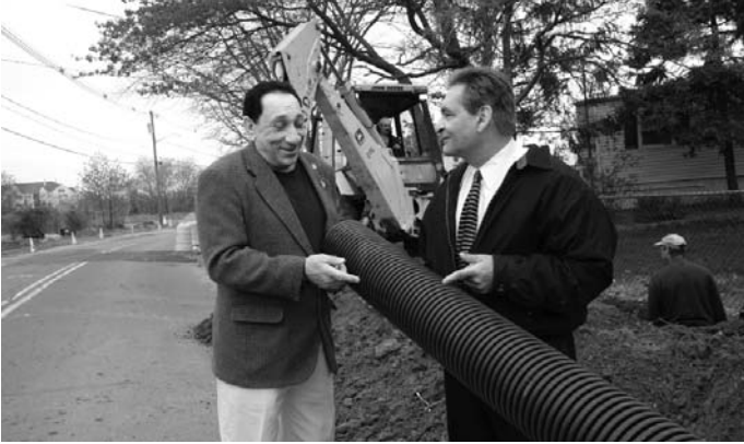
Director of Public Works Jim Lauro (r.) shows Councilman Vincent Vinci piping being installed under Gerard Ave. as part of road reconstruction.
